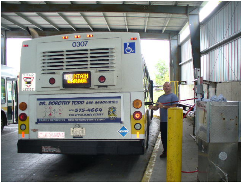
CNG bus refuelling at HSR bus garage
